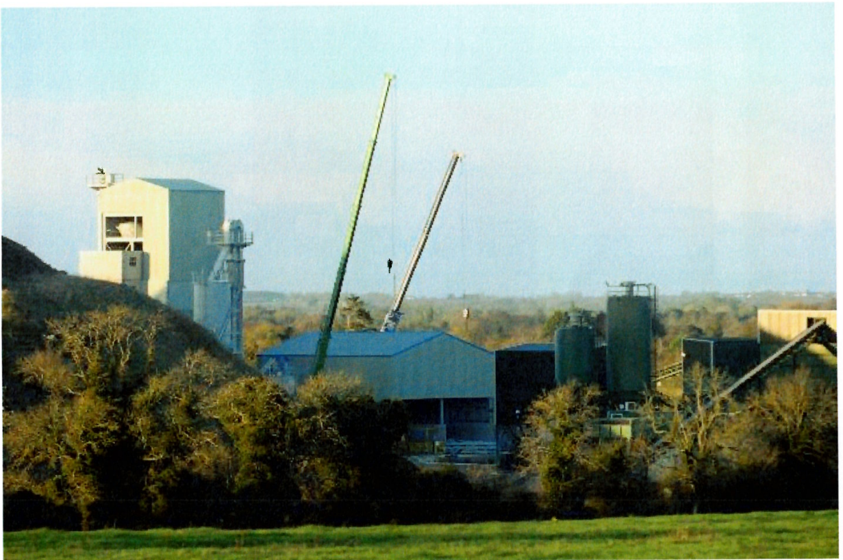
Construction of plant in 2016 without planning consent
